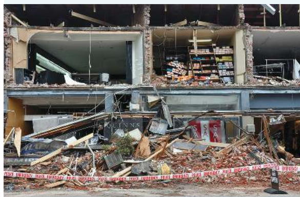
FIGURE 8.63 Damage caused by the 1989 Newcastle earthquake
