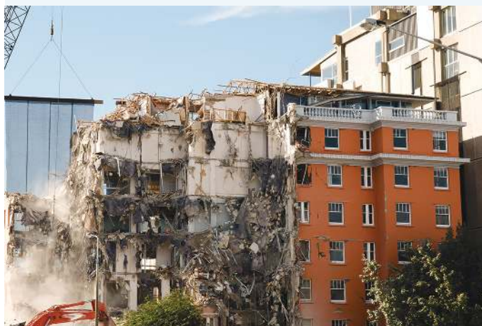
FIGURE 8.37 In February 2011, a magnitude 6.3 earthquake struck Christchurch, New Zealand. The earthquake destroyed many buildings and homes, injured thousands, and killed 185 people.
