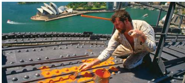
FIGURE 6.25 The Sydney Harbour Bridge is continually painted to protect it from moisture and the air, which would cause its steel girders to rust.
