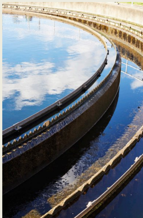
FIGURE 2.3.2 During secondary wastewater treatment, bacteria help break down solids and clean the water. Cleaned water overflows around the rim of the tank, from where it is channelled off for more treatment.
