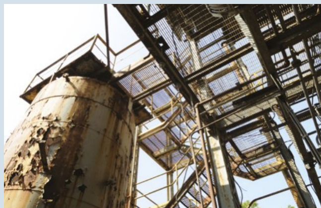
FIGURE 17.1.18 Over thirty years after the Union Carbide disaster, the site remains in a dilapidated and contaminated state.
