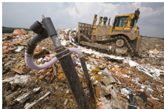
FIGURE 12.2.14 Pipes buried in this rubbish tip collect biogas.
