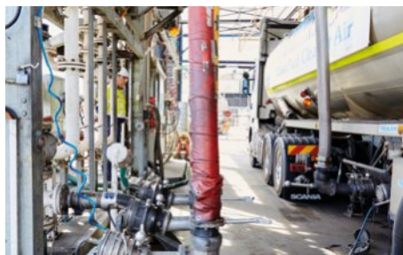
FIGURE 17.1.7 A tanker loads bioethanol at Manildra. The plant is located near the wheat processing facility.
