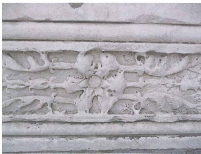
Figure 43.3 Pitting in marble due to acid rain (Pisa, Italy).
