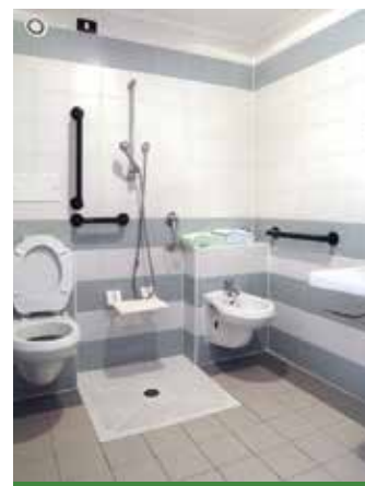
Figure 5.8 Safety instalments in a bathroom.
