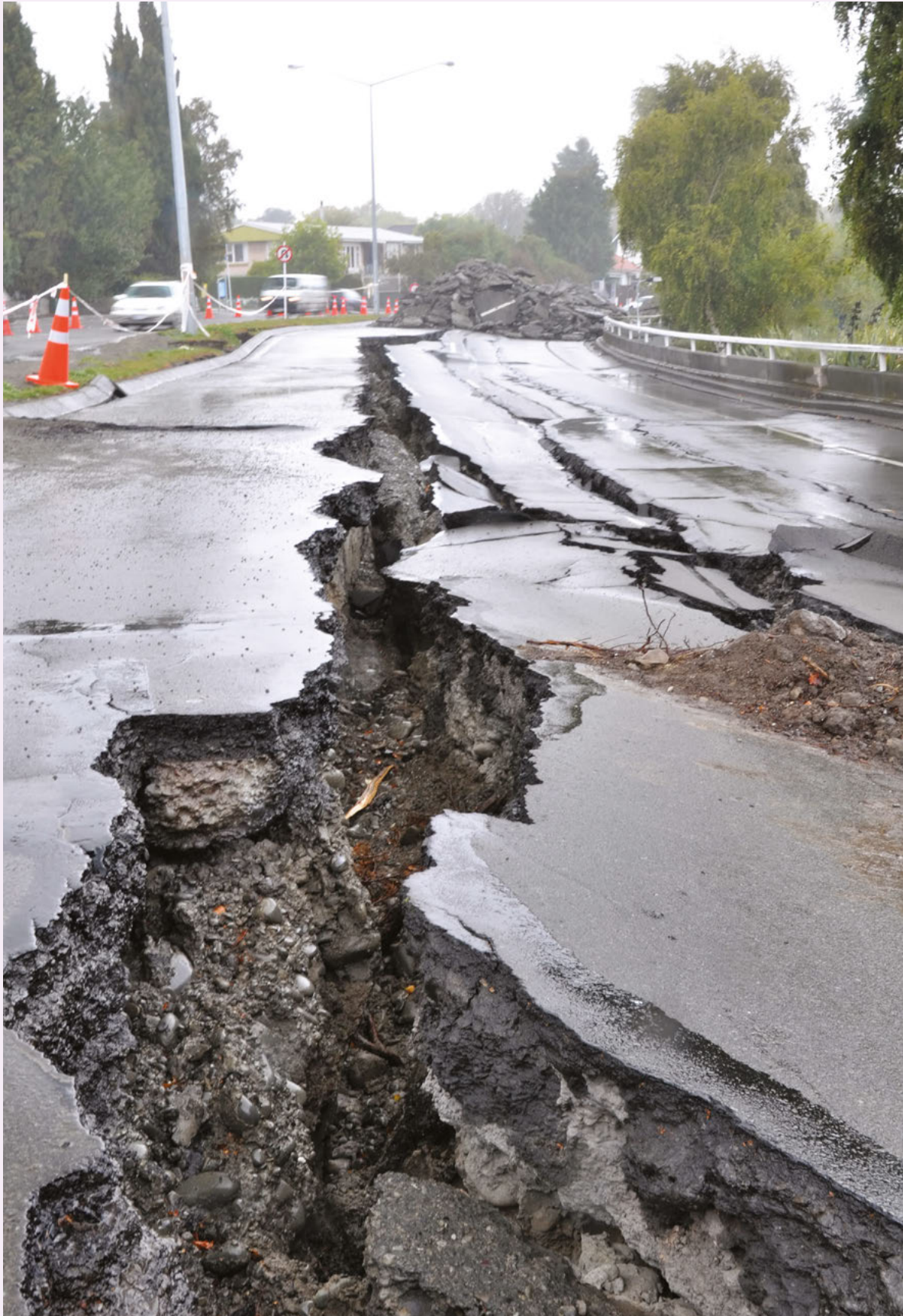
Source 5.14 A seriously damaged road in Christchurch, New Zealand, after the earthquake of 2011 which measured 6.3 on the Richter scale
