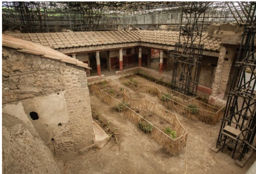
FIGURE 14.21 The extensive work on the restoration of the House of the Tragic Poet at Work
