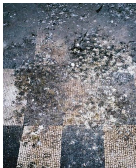
FIGURE 13.5 Destruction by pigeon droppings
