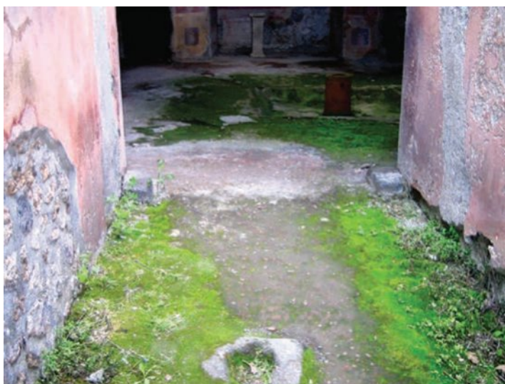
FIGURE 13.4 The effect of water pooling on floors
