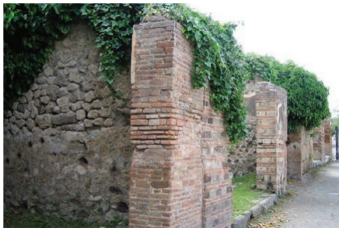
FIGURE 14.8 Rampant ivy clinging to walls
