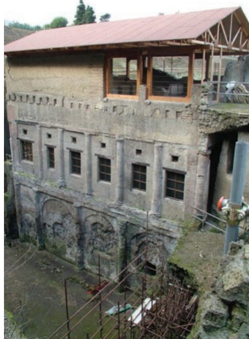
FIGURE 13.12 Protective roofing, stabilisation and exposure of lower level of the House of the Relief of Telephus in Herculaneum
