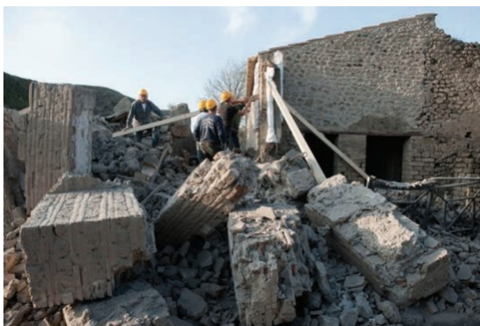
FIGURE 14.1 The collapse of the Schola Armaturarum
