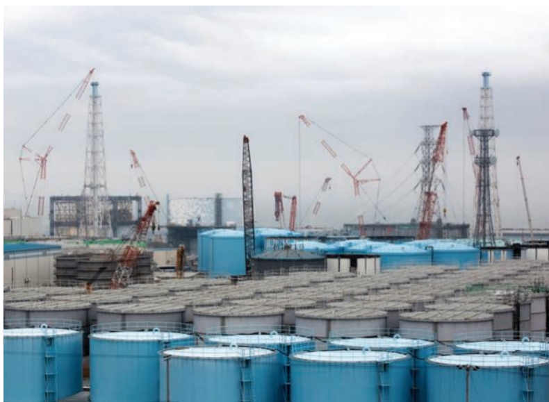
SOURCE 12.64 The closing down and clean-up under way at the Fukushima Daiichi Nuclear Power Plant in north-eastern Japan, following a powerful earthquake and tsunami on 11 March 2011. The tanks in the foreground are some of more than 900 that have been built to store water contaminated with radioactive material. This includes both water used to cool the reactors and groundwater contaminated by leaks from the reactors. The clean-up is estimated to take 30 to 40 years.
