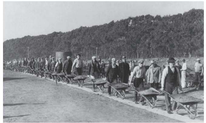
SOURCE 6.51 Workers on their way to fill a gully with wheelbarrows of earth during the construction of a major road, under President Roosevelt's New Deal, San Francisco, California, 1934
