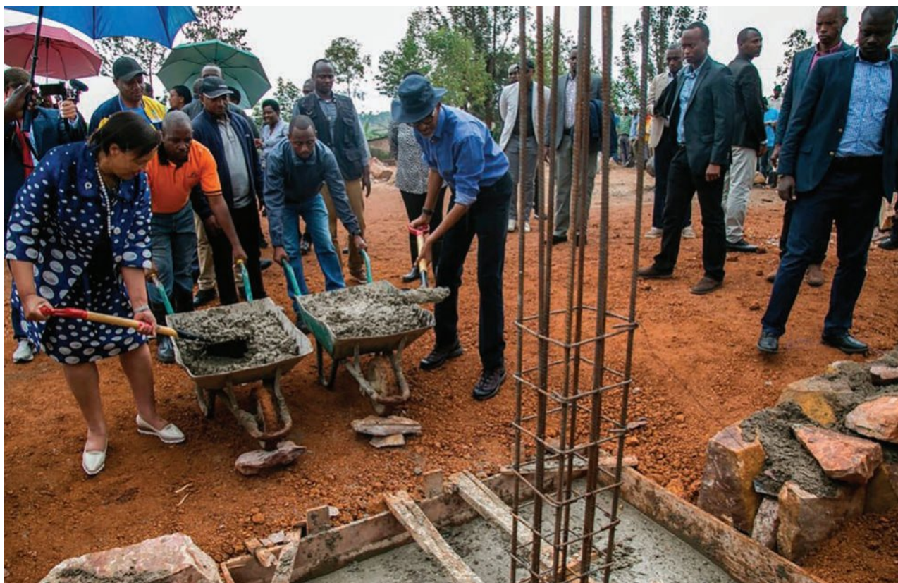
Figure 5.22 President Paul Kagame and Commonwealth of Nations Secretary General Patricia Janet Scotland take part in the monthly umuganda by scooping concrete on the construction site of a secondary school in Gahanga district in Kigali.
