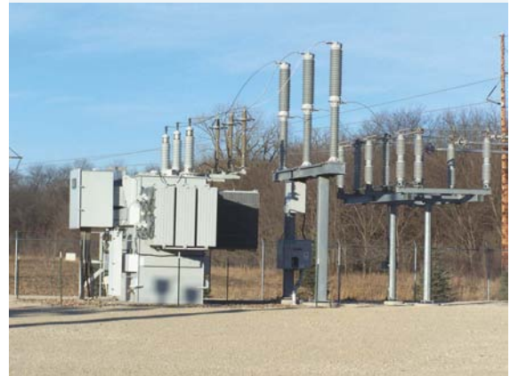
FIGURE 6.26 A transformer at a substation.
