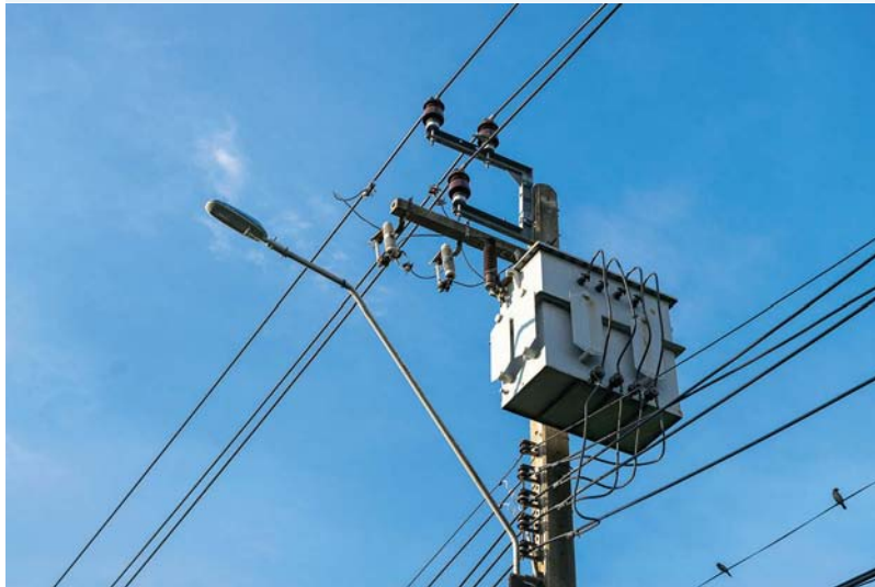
FIGURE 6.27 A pole transformer.
