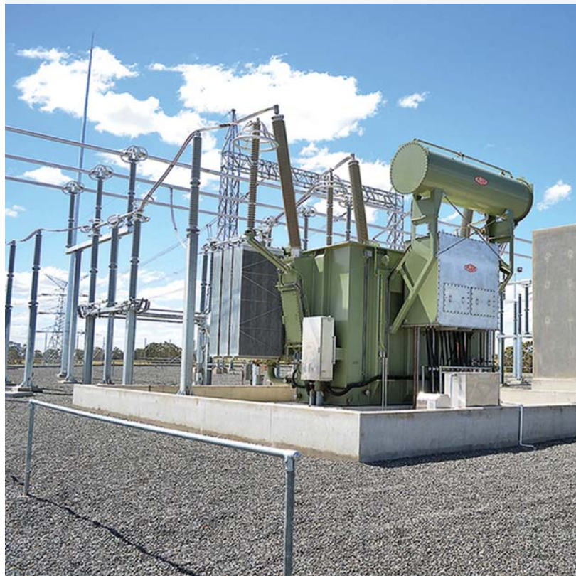
FIGURE 6.1 A large 90MVA 330/33KV power transformer for a windfarm and powerlines, located in NSW.
