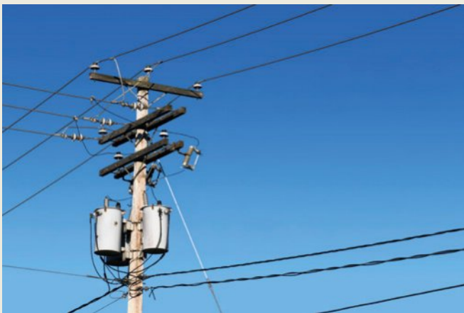
FIGURE 14.2.15 Electric power line poles carry the current and power to houses, hold transformers (grey boxes), and sometimes carry telephone cables.
