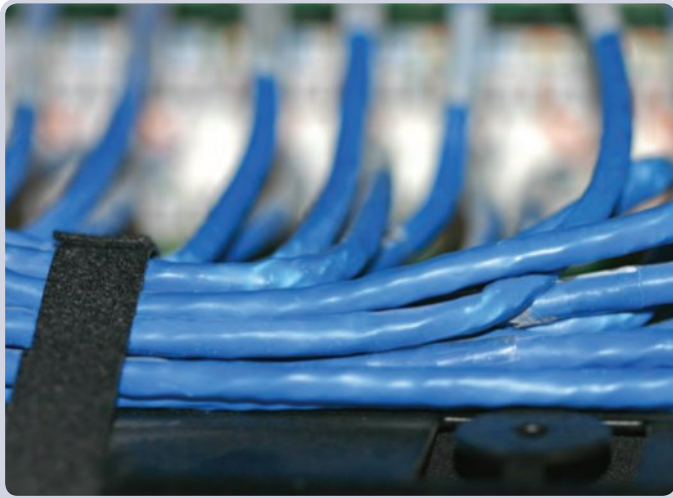
Figure 7.28 Network connection cables join hardware
