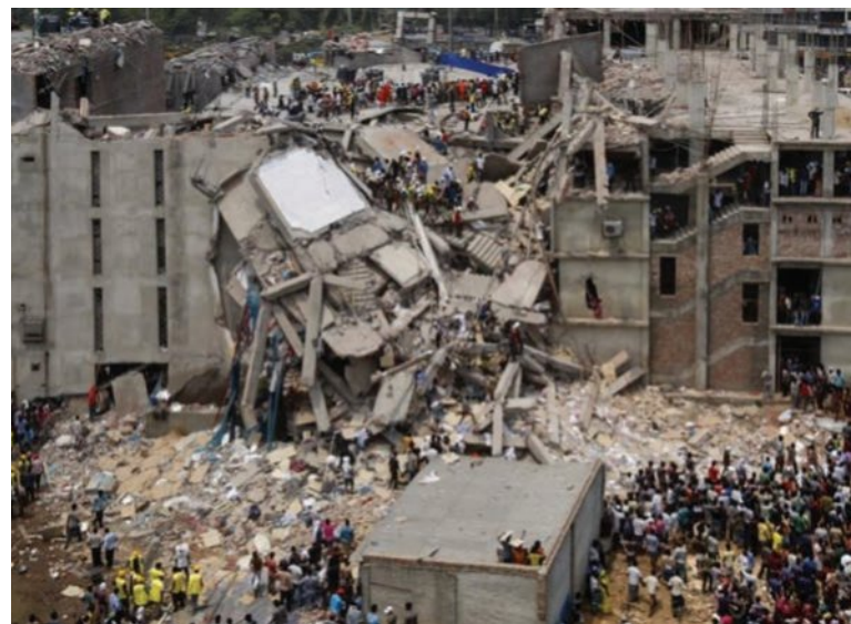
▲ Figure 13.9 On 24 April 2013, the eight-storey Rana Plaza in Dhaka, Bangladesh, collapsed. The death toll was 1134 people.
