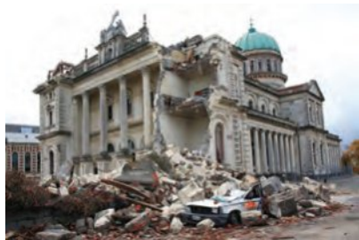
Figure 4.9b This is a damaged Catholic Cathedral. The earthquake of 2011 killed 185 people and damaged thousands of buildings in Christchurch.
