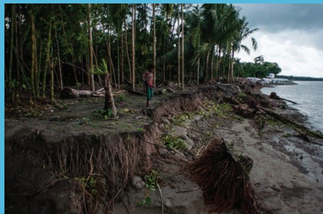
▲ Figure C Erosion of a bank of the Meghna River, Bangladesh
