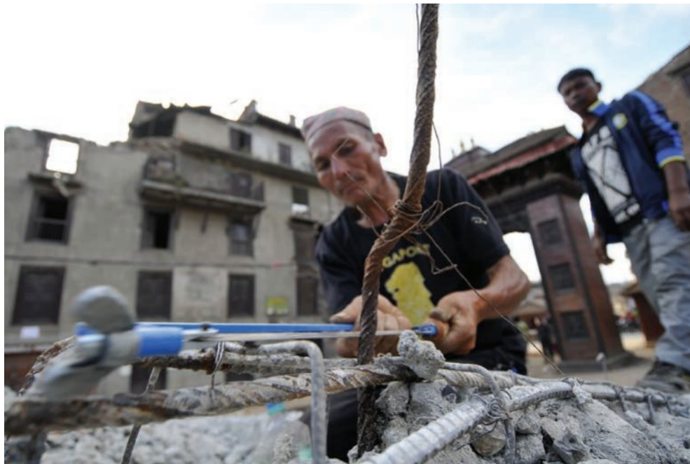
▲ Figure 4.117 Gyan Binayak Phateja, 50, helps his neighbour by cutting iron rods from collapsed structures at Thulo Byasi in Bhaktapur, Nepal on May 14, 2015.
