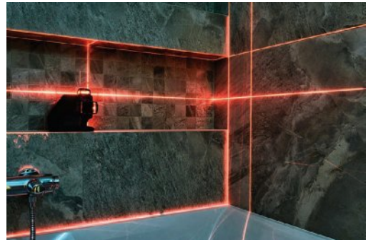
Modern measuring tools include lasers, being used here to check measurements in a bathroom.
