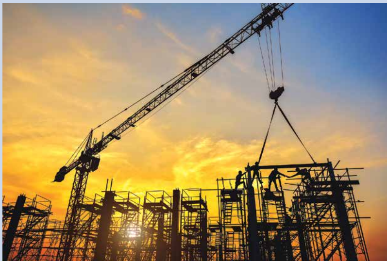
Construction material moved onto a building by a modern crane has undergone a combination of transformations.
