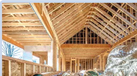
A builder makes sure that the roof rafters are all parallel, the ceiling joists are horizontal and parallel, and the wall studs are perpendicular and parallel.
