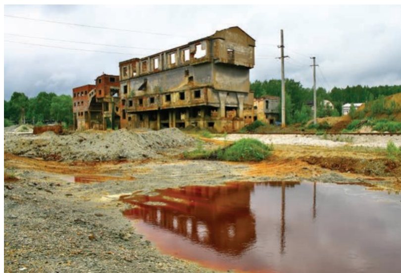
Figure 8.10 The orange toxic water produced here is due to the reaction of acid rain with the metal in this abandoned mine.
