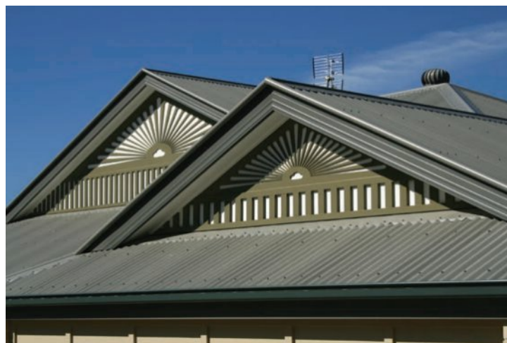
Figure 8.17 A galvanised corrugated-iron roof: the zinc coating will corrode before the iron underneath, preventing rusting of the iron.
