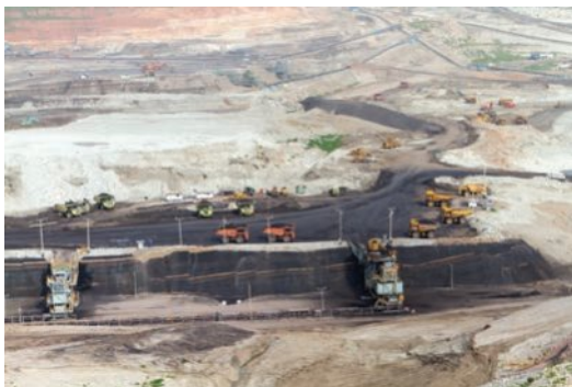
Figure 5.91 Constructing a mining site involves many people, such as construction workers, builders, landscape architects and engineers.
