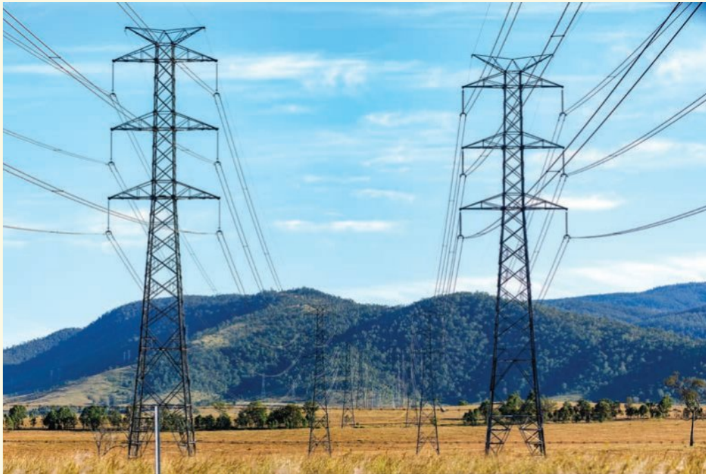
Figure 6.11 Transmission lines deliver electrical energy to all parts of Queensland, losing a minimal amount as heat.
