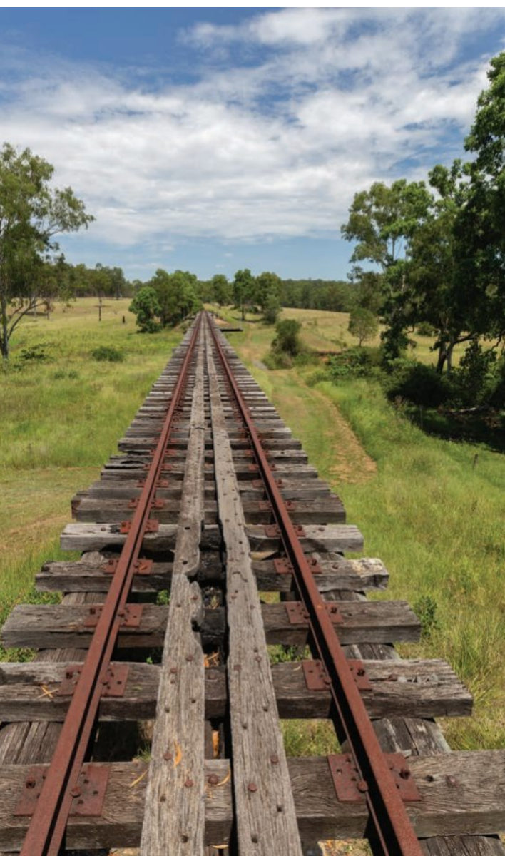
Figure 8.26 The rusting on a railway track is evidence of a chemical reaction.
