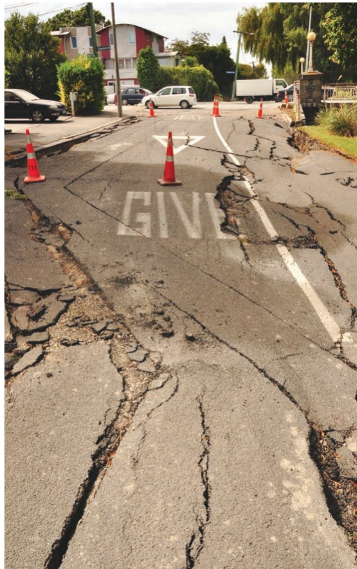
Figure 6.5 The energy of an earthquake damaged this road in Christchurch, New Zealand, in 2011.
