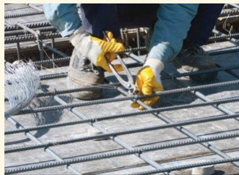
Figure 4.74 To make concrete more suitable for seismic activity, engineers add steel (in the form of rebar), which is much more flexible.
