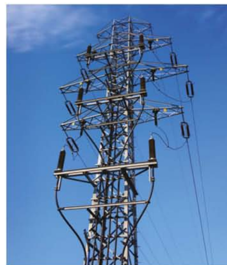
FIGURE 3.1.2 This power transmission tower relies on the strength of iron in steel for its structural integrity. The electricity cables are made from aluminium, utilising its ductility and electrical conductivity.
