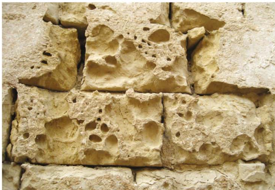
FIGURE 20.1.5 The cavities in this limestone wall have been corroded by acid rain.
