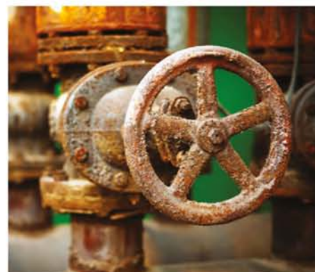
FIGURE 16.3.1 Corrosion is causing water to leak in these pipes in a pumping system.
