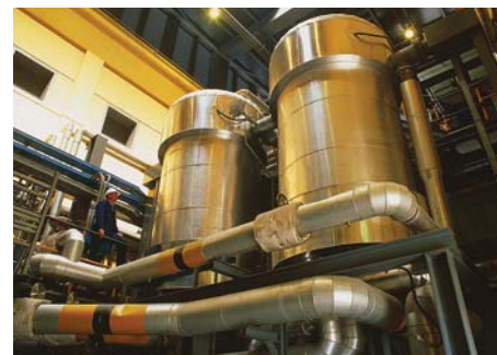
FIGURE 6.1.9 Interior of the PRODE fuel cell power station in Milan, Italy, which began operating in 1992. The cells use hydrogen as the fuel and phosphoric acid as the electrolyte. The fuel cells can produce up to 1.3 MW of electricity.
