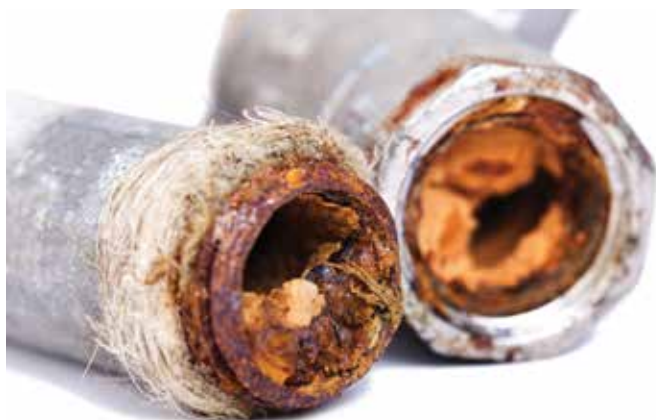
Scale inside steam pipes can be avoided by altering the pH of the water.
