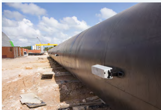
FIGURE 14.14 Sacrificial anode for cathodic protection on a pipe
