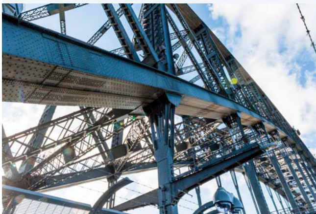
FIGURE 3.20 Exposed surfaces on the Sydney Harbour Bridge must be repainted every five years. But with a surface area of nearly 500 000m 2 , painters are permanently employed to ensure that the Sydney Harbour Bridge is protected against corrosion.
