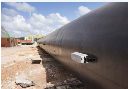
FIGURE 12.16 Sacrificial anode for cathodic protection on a pipe
