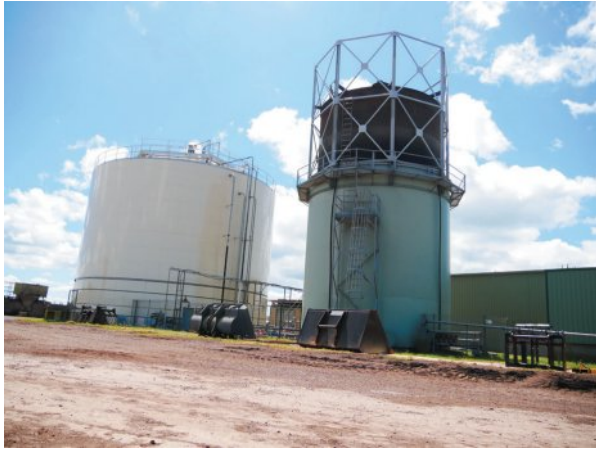
Bioenergy digester on Berrybank Farm
