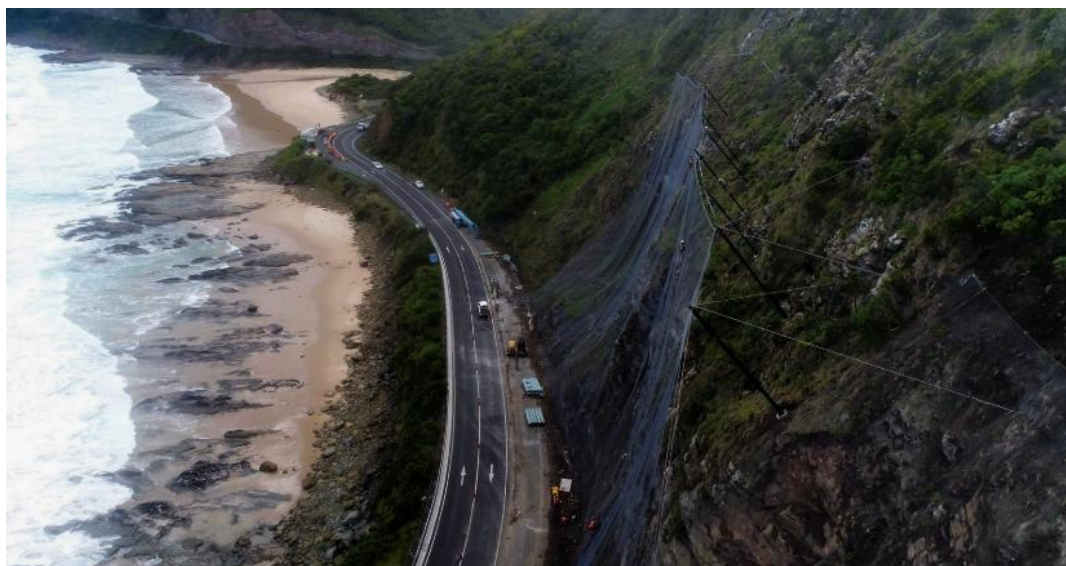
◀ Figure 7.6 An attenuator used to stabilise the 160 metre cliff face at Cumberland River on the Great Ocean Road
