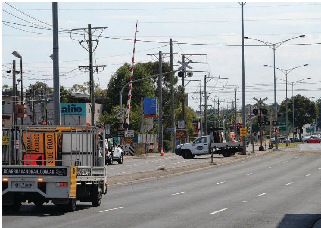
◀ Figure 7.2 Level crossing maintenance on Bell Street, Preston where high levels of traffic congestion occur
