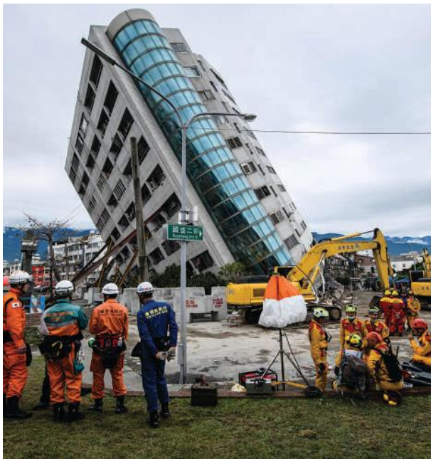
▼ Figure 3.20 Rescue services search for people in a damaged building in Hualien, eastern Taiwan, 9 February 2018
