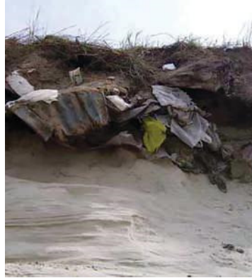
▼ Figure 4.31 The erosion of dunes covering two closed landfill sites in the northeast of East Beach are posing a land contamination risk
