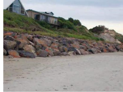
▼ Figure 4.32 The existing rock seawall on East Beach has been repaired and upgraded to protect the dunes from erosion
