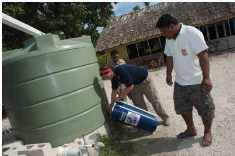
FIGURE 13.29 The installation of water tanks provides Kiribati with clean water that is not contaminated by seawater during floods and king tides due to climate change.
