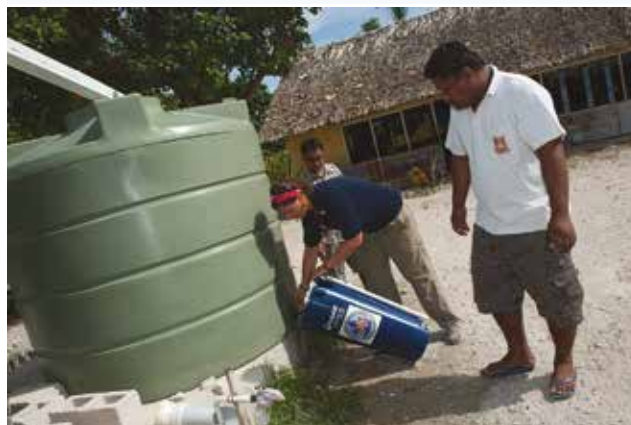
FIGURE 13.39 The installation of water tanks provides Kiribati with clean water that is not contaminated by seawater during floods and king tides due to climate change.
