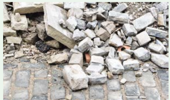
Source 2 In 2014, a brick wall in Brighton East collapsed during strong winds, killing Michael Klanja.
