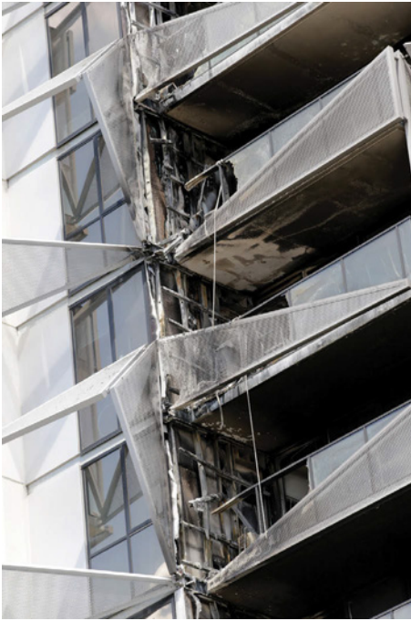
Source 3 The Lacrosse tower was extensively damaged by the fire.
