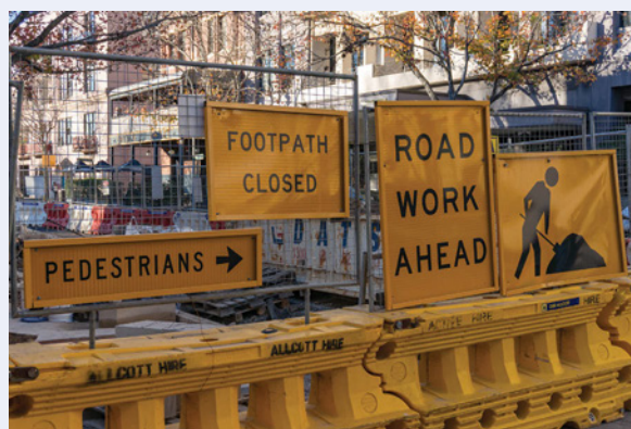
Source 3 Work on Melbourne's Metro Tunnel generates medium-level noise, with periods of high-level noise during excavation and work on retaining walls. Where possible, high-impact work is undertaken during the day, although this is not always possible. Tunnel works have also made parking severely limited in some areas.
