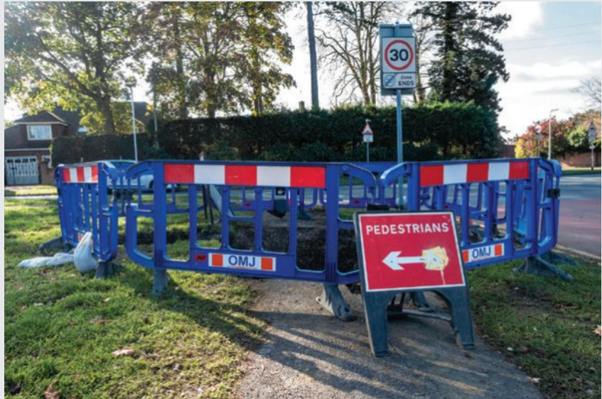
Source 4 Barriers are sometimes used to ensure people are not injured from works on pathways and roads
