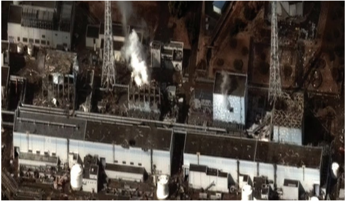
Figure 4B–5 The Fukushima Daiichi Nuclear Power Plant disaster caused damage to the buildings housing reactors 1–4. The visible damage was caused by explosions of hydrogen gas released by the reaction of hot zirconium alloy with steam from the steam generators. Inside, the cores of reactors 1 and 2 have melted and pooled at the bottom of their concrete containment vessels. The cause of the disaster was the 2011 Tōhoku earthquake and tsunami that destroyed the emergency generators powering the reactor cooling pumps, leading to the reactors overheating.
