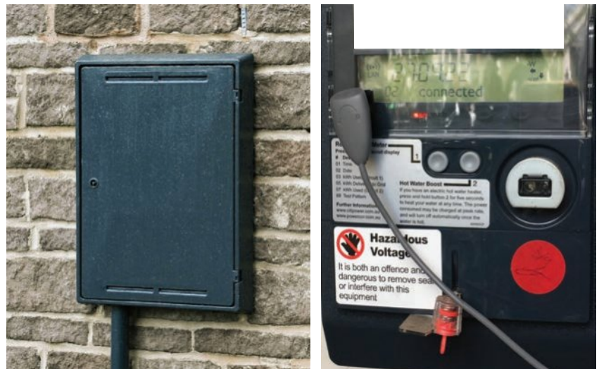
Figure 6B–6 Meter box (left) and a ‘smart’ meter (right) can be read remotely as well as on-site. This meter has a PowerPal attached, which measures the power consumed in real time and relays it via Bluetooth to a phone app, which allows a view of total energy consumption through the day and also an estimate of the cost.
