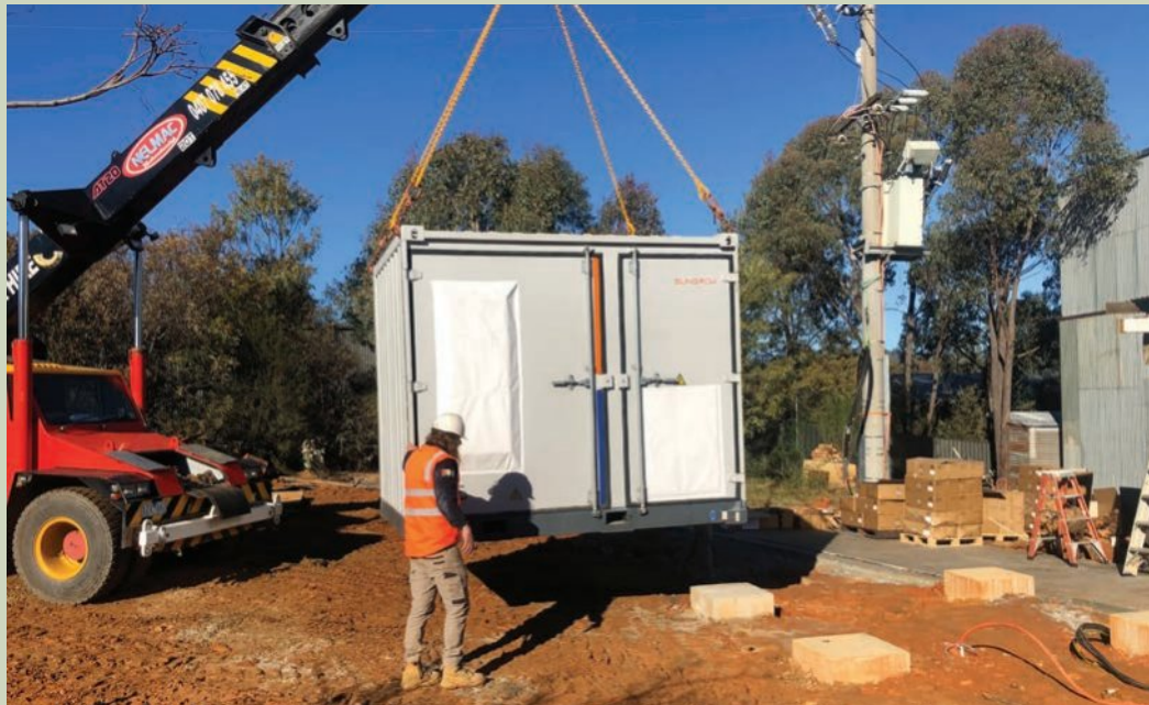
Figure 6C–1 TRY community battery being craned into position in June 2021. The battery – which was Victoria's first behind-the-meter, community-owned solar-and-battery system – now stores solar energy from a 64 kW solar array. It has the capacity to power up to 40 Yackandandah households, including through the evening peak.
