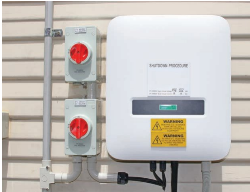
Figure 5A-5 An inverter for a domestic solar panel installation, with isolating switches
