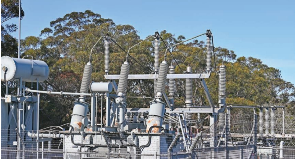
Figure 6C–4 A substation with step-down transformers to convert HV (high-voltage) AC, such as 200 kV, to lower voltage, 415 or 230 V, for distribution to local houses and businesses.
