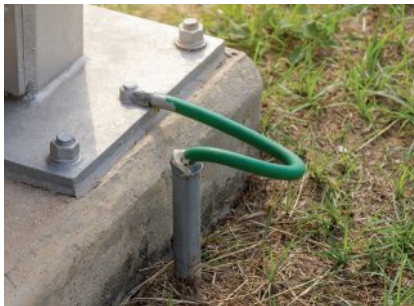
Image: TS Photographer/Shutterstock.com Figure 7 Earth wires are connected to the ground (the earth).
