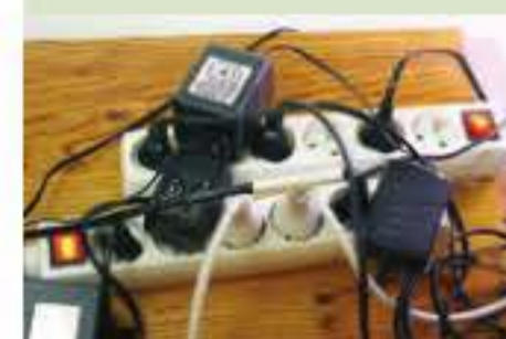
Overuse of power boards and double adaptors can cause overloading of circuits. This can cause wires and components to overheat and start a fire.
