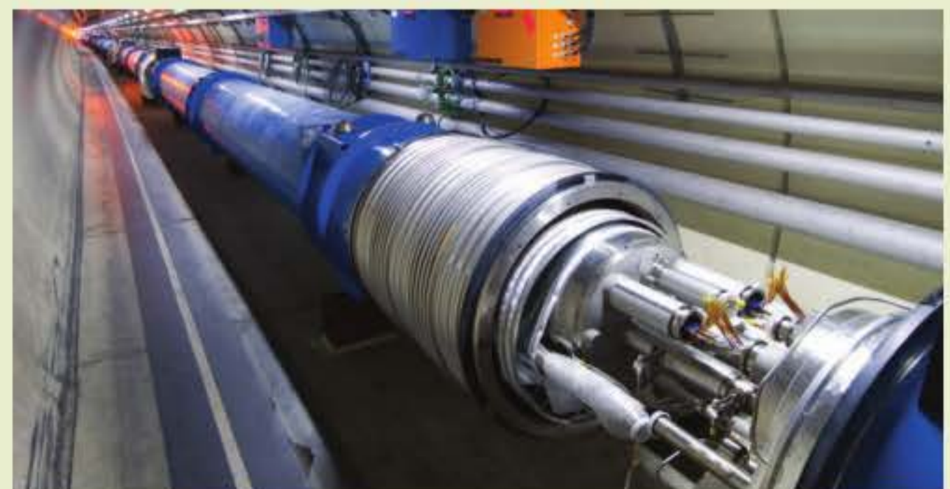
FIGURE 9.1.14 Two LHC magnets before connection. The blue cylinders contain the magnets and a liquid helium system that cools them so they become superconducting.
