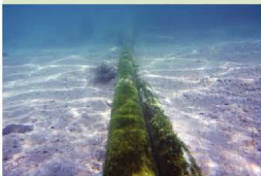
Underwater cables form the backbone of the internet.
