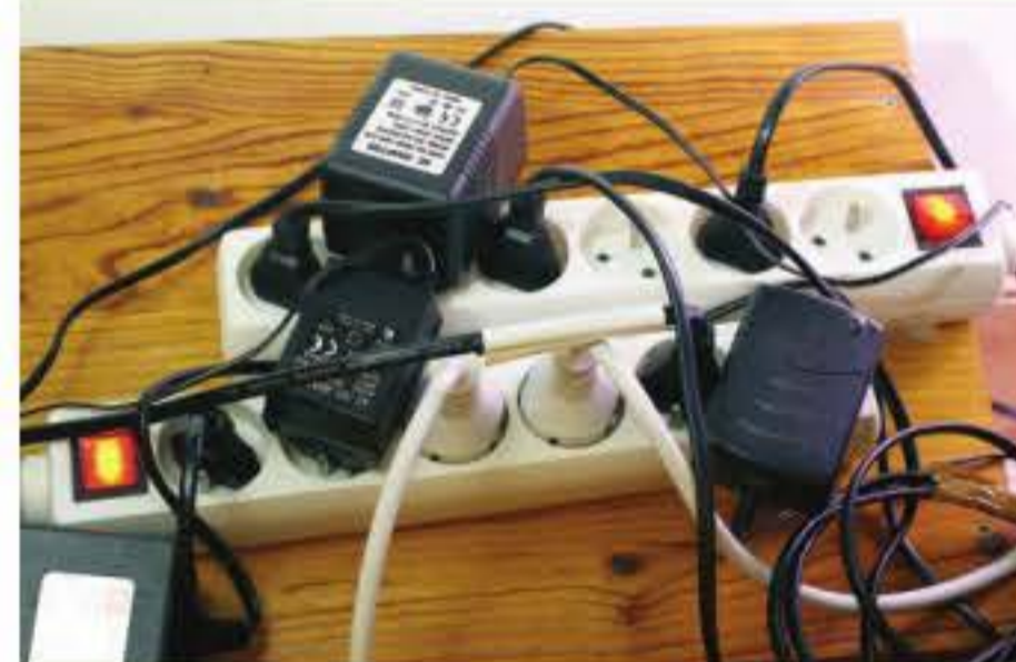
Overuse of power boards and double adaptors can cause overloading of circuits. This can cause wires and components to overheat and start a fire.
