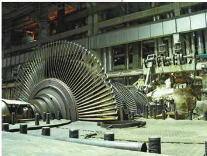
Vanes of a turbine at a coal plant
