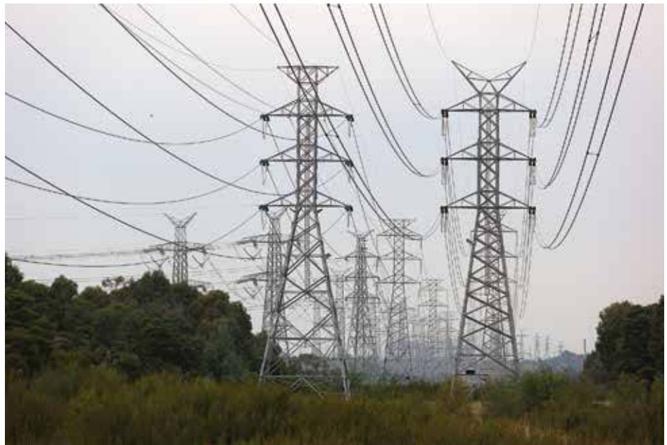
Transmission lines and towers near Melbourne
