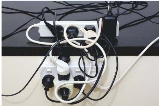
FIGURE 7.12 Overloading of an electric circuit
