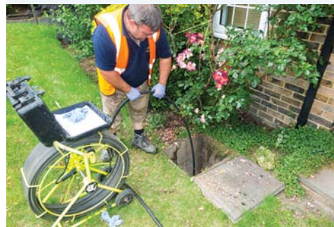
FIGURE 2.16 Fibre optic cable with a camera used to investigate a blockage in a pipe
