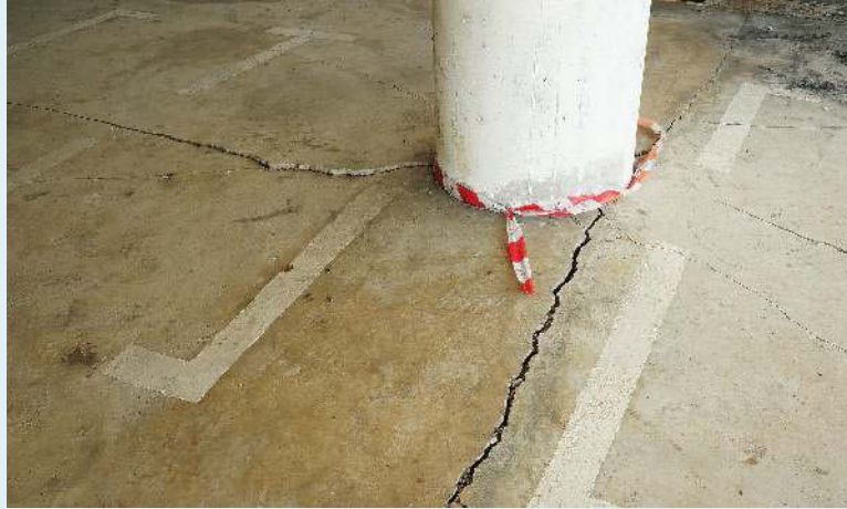
FIGURE 11.4.14 A cracked concrete floor resulting from tensile stresses
