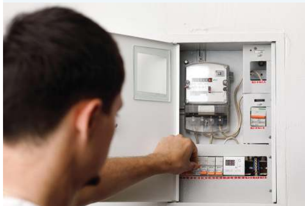
FIGURE 7.3 Many houses have a meter and circuit breaker in their meter box. The circuit breaker is in the bottom left corner.
