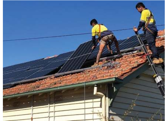
FIGURE 6.25 Solar panels are connected together in a rooftop array.
