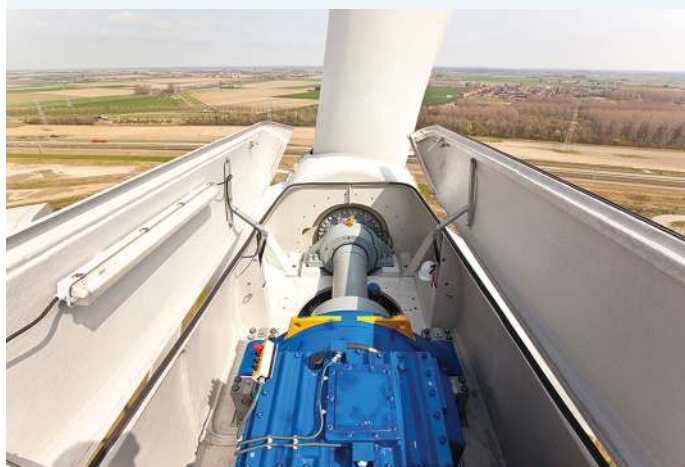
FIGURE 6.1 A generator inside a wind turbine
