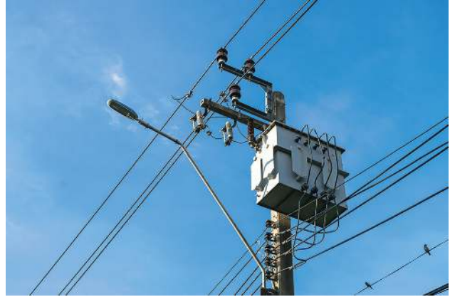
Figure 7.9 A pole transformer
