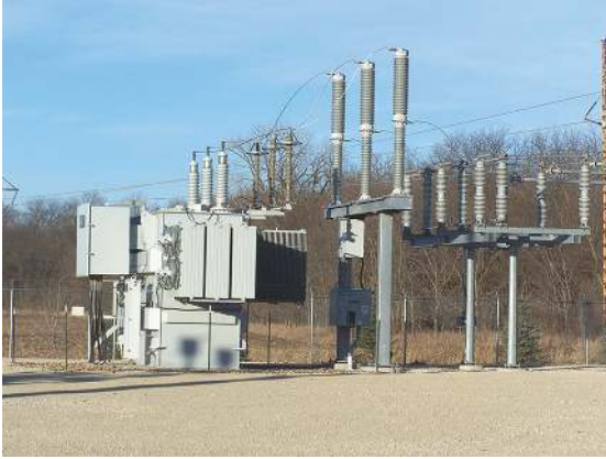
Figure 7.8 A transformer at a substation
