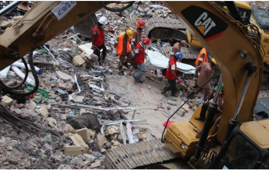
Figure 1.9 Rana Plaza building collapse, 2013
