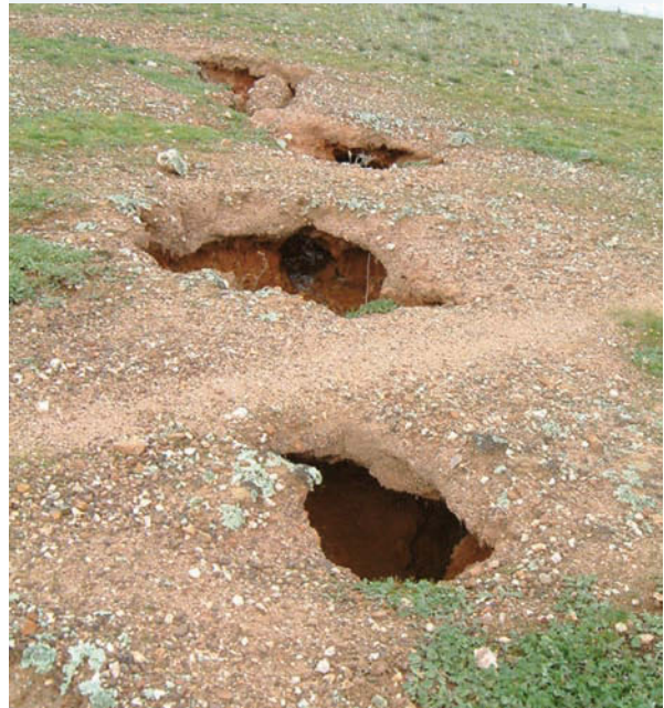
FIGURE 5 Tunnel erosion. What do you notice about the ground around these tunnels? What do you think will happen if water flows through them?
