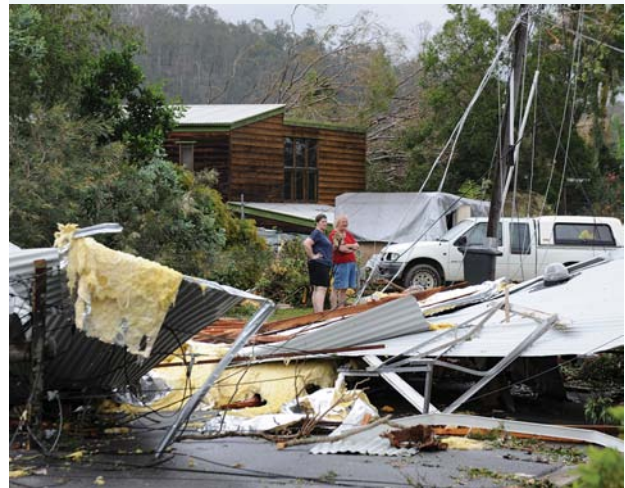
FIGURE 10 The roof of a house sits in the middle of the road at The Gap in Brisbane's north-west. The roof is from a home 50 metres away.
