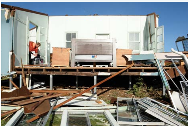
FIGURE 13 Structural damage in Yeppoon
