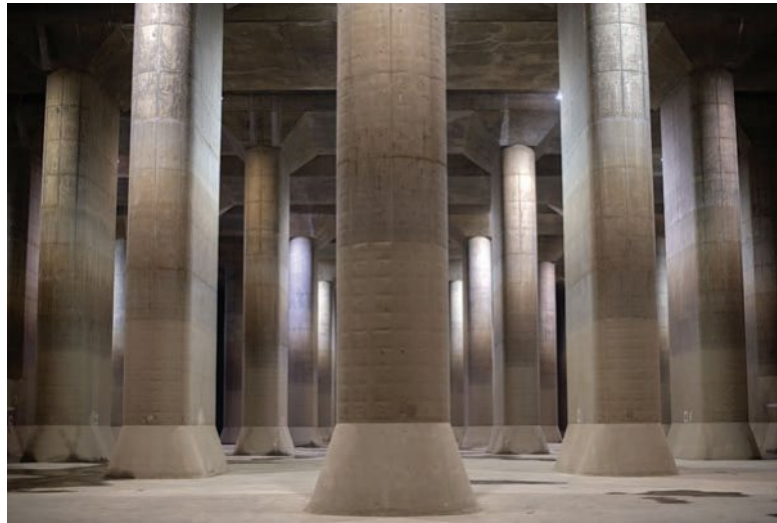
▲ Figure 9.28 Tokyo's Metropolitan Area Outer Underground Discharge Channel
