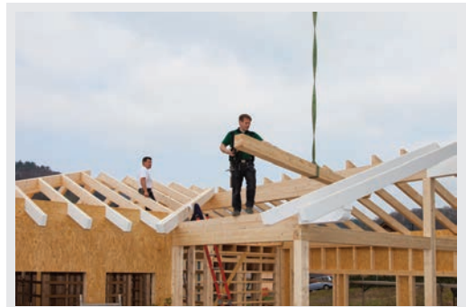
To calculate the number of rafters needed to support a roof, a carpenter first divides the roof span (its length) by the required space between each rafter.
