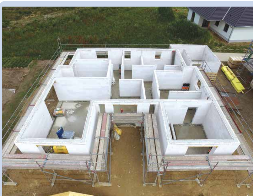
The perimeter of a house is found by adding the lengths of all the outside walls. Scaffolding is required around the perimeter for construction work above ground level.
