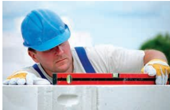
A builder uses a spirit level to check that bricks are horizontal
