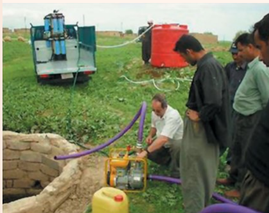
FIGURE 7.30 A water purification system in Kendala
