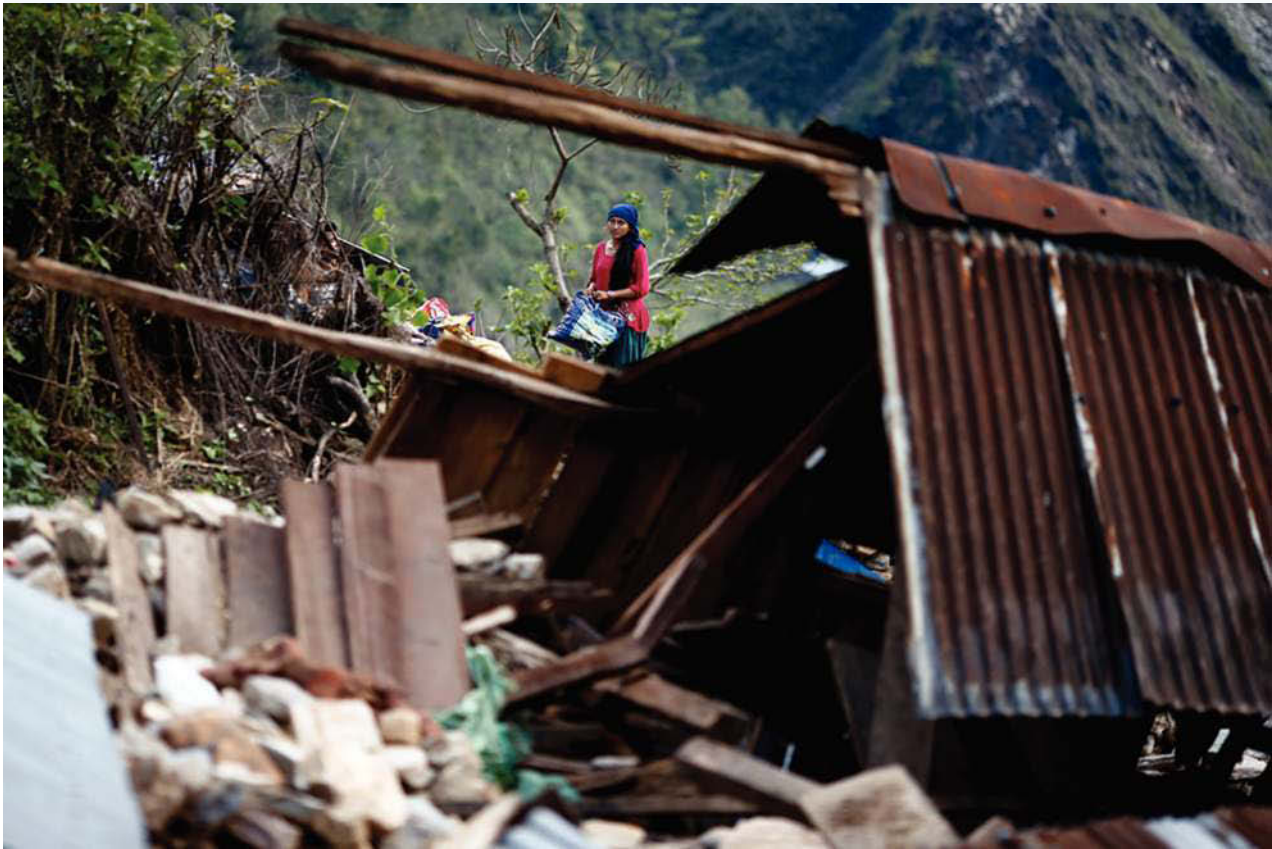
FIGURE 14 Compared to some richer countries, such as Japan and the United States, very few buildings in Nepal are earthquake-proof.
