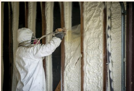
FIGURE 9.15 A worker spraying closed cell spray foam insulation between the timbers in a wall
