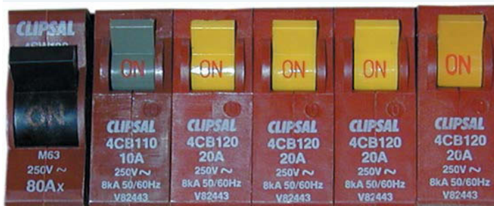
FIGURE 10.57 The switch on the left is a safety switch. The other switches are circuit breakers.
