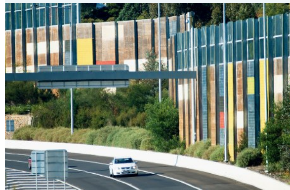
FIGURE 9.36 The effect of freeway noise on nearby residents is reduced by barriers that absorb and reflect sound energy.
